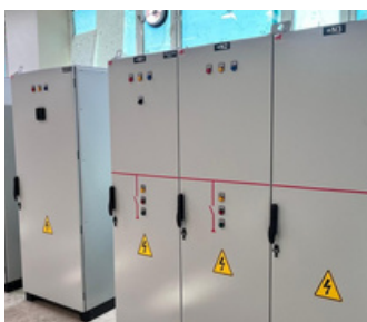
LV SWITCHGEAR PANELS ALL Low Voltage Systems.
