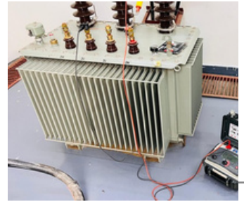
TRANSFORMERS Low Voltage Systems.
