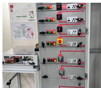
DISTRIBUTION BOARDS ALL Low Voltage Systems.
