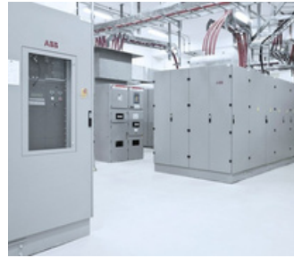
DISTRIBUTION SUBSTATIONS Medium Voltage Systems.
