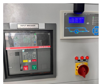
AUTOMATIC CHANGE OVER SYSTEMS ALL Low Voltage Systems.
