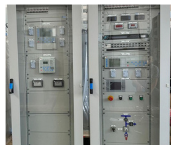
SCADA & PROTECTION SYSTEMS ALL Low Voltage Systems.
